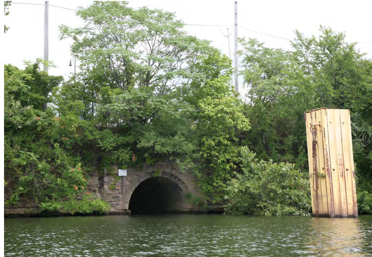
Combined sewer overflow
